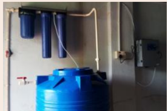
Three safe water systems were installed in the state of Andhra Pradesh, in the month of October.
