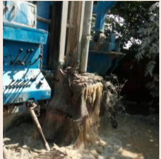
A new bore well was installed at Faith Baptist Orphanage in Savakanahalli, Bangalore. The water was found at a depth of 1265 feet.
